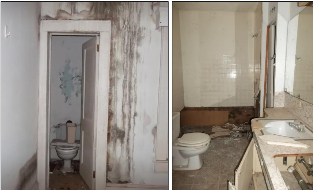
Photo 64: Looing East in the Half Bath (Left) and Full Bath (Right) in the Ell.
