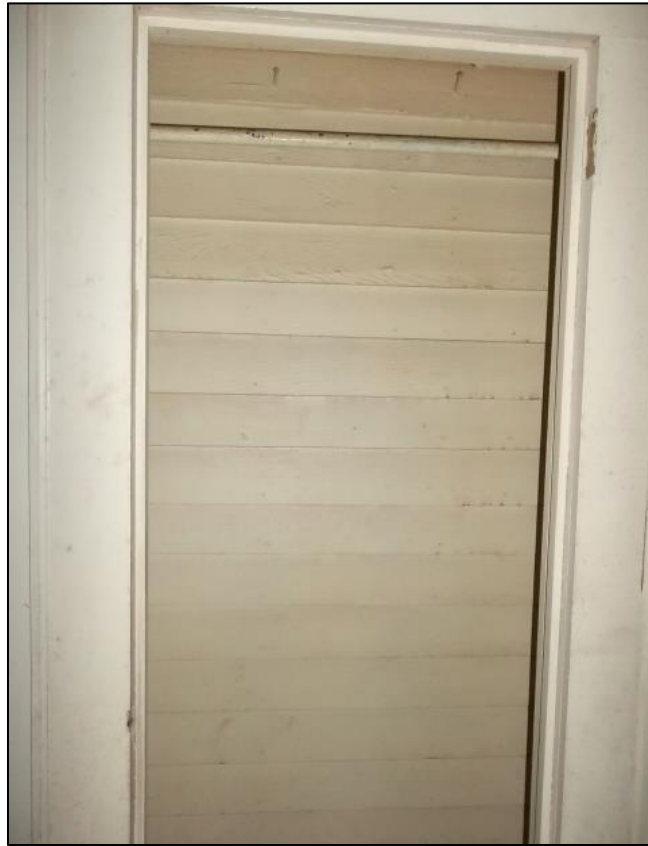
Photo 62: View of the Weatherboard at the Back of the Closet in the Southeast Room.
