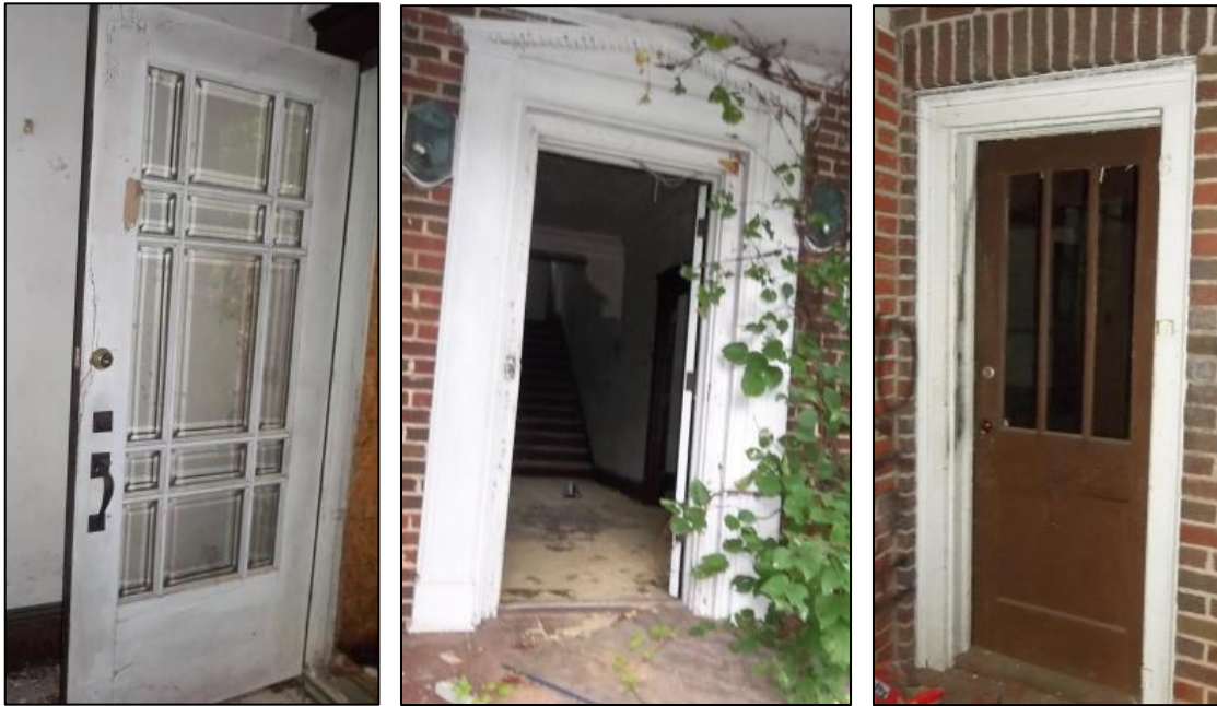
Photo 8: Doors at the R.O. Caldwell House. The primary entrance door on the east elevation (left), primary entrance door frame (center), rear-elevation door (right).
