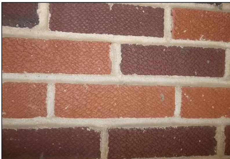
Photo 41: Detail of the Textured Bricks Used on the Exterior of the House.
