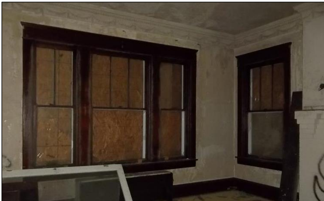
Photo 9: Original Windows on the R.O. Caldwell House, Looking at the Southeast Corner.
